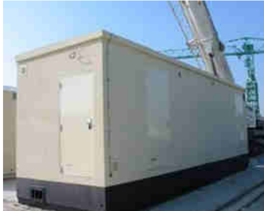
Example of substation
